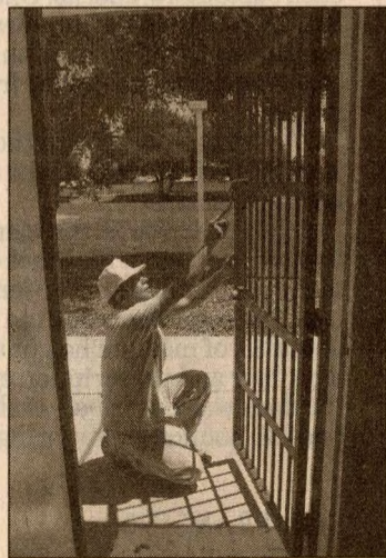
Hassan Naddaf of Mountain View works on restoring the restrooms at Farrell Park.
